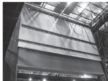
Straight Lift Fire Curtain
